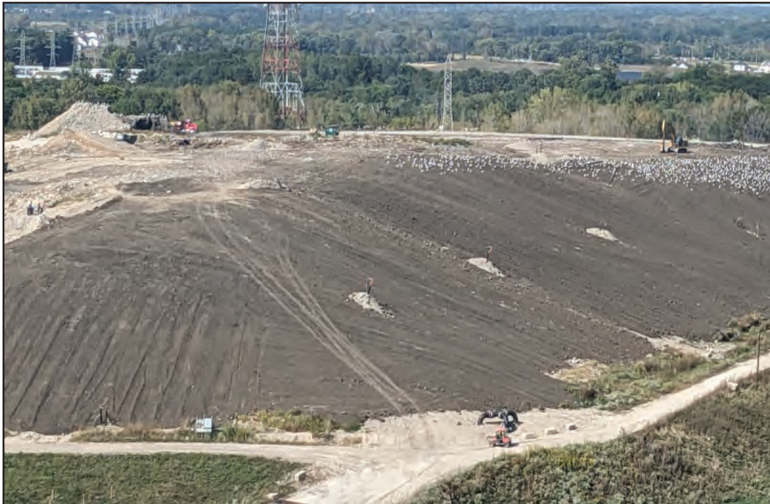
Phase 1 & portion of 2 with top soil cover to grow vegetation, reduce erosion and dust
